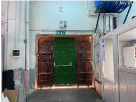
Emergency Exit Door.jpg
